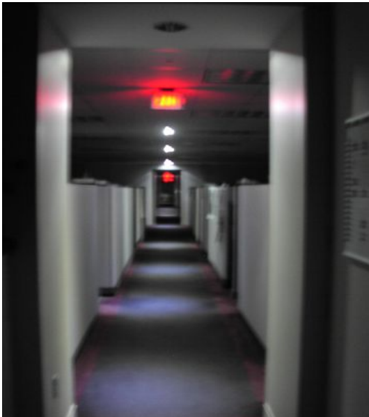
IN THIS HALLWAY POWER USE WAS REDUCED BY ABOUT 3,000 KWH PER YEAR
